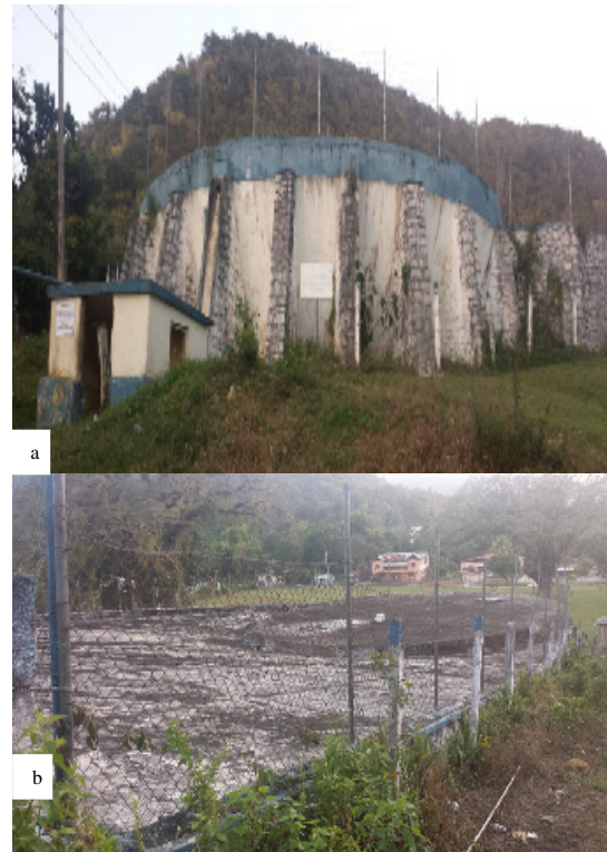
Fig.5. (a) An elevated rainwater concrete catchment of Elisabeth, Jamaica; (b) the surface runoff and the storage tank of Elisabeth, Jamaica RHI
